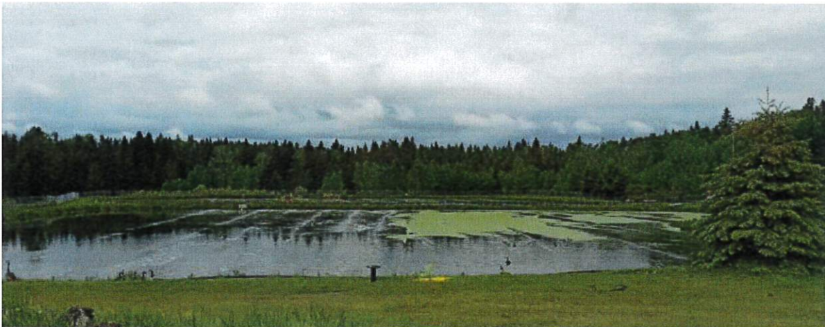
Figure 1. Can-Air linear bubble airline (left) compared to competitors' bubble airline (right) installed in the Village of Caroline, AB wastewater lagoons.
